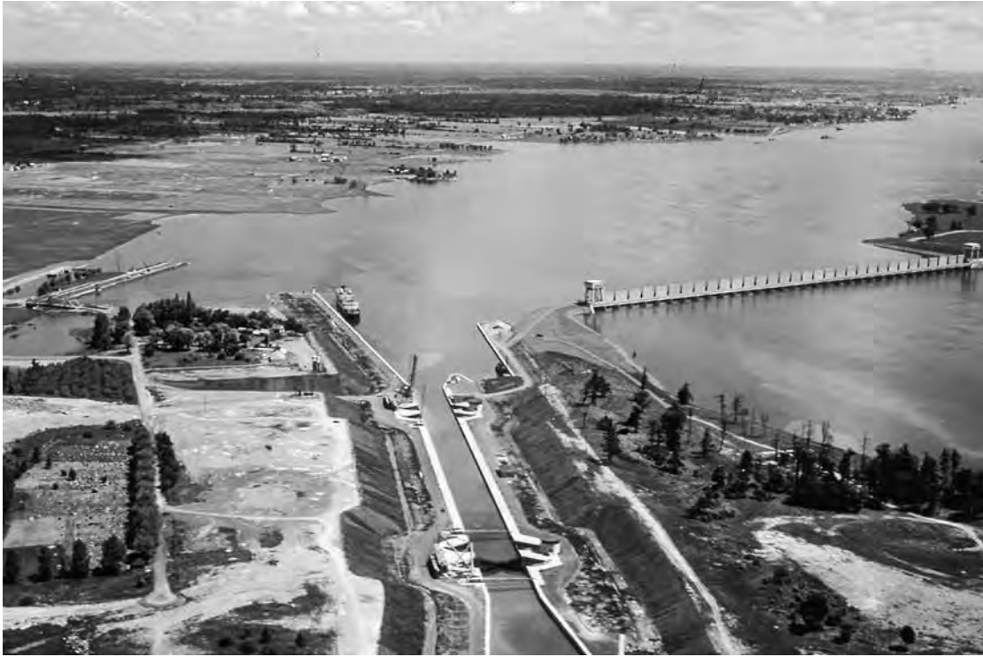
FIGURE 0.6 Iroquois Lock and Control Dam during construction (the old lock and canal can be seen to the left). © Dumas Seaway Photograph Collection, Mss. coll. 124, Special Collections, St. Lawrence University Libraries
