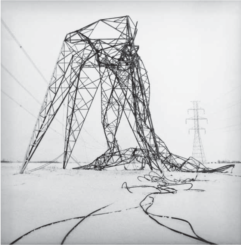
FIGURE 11 Benoit Aquin, “Le verglas #16, Boucherville” (1998). This stunning photograph of a collapsed power line, caused by the ice-storm that struck areas of south-central Canada during the winter of 1998, was part of the photo-essay “Lethal Beauty,” by Montreal photographer Benoit Aquin. It provides a striking reminder of Canadian nordicity and of the vulnerability of our technologically sophisticated society. Reproduced with the artist’s permission. © Benoit Aquin.
